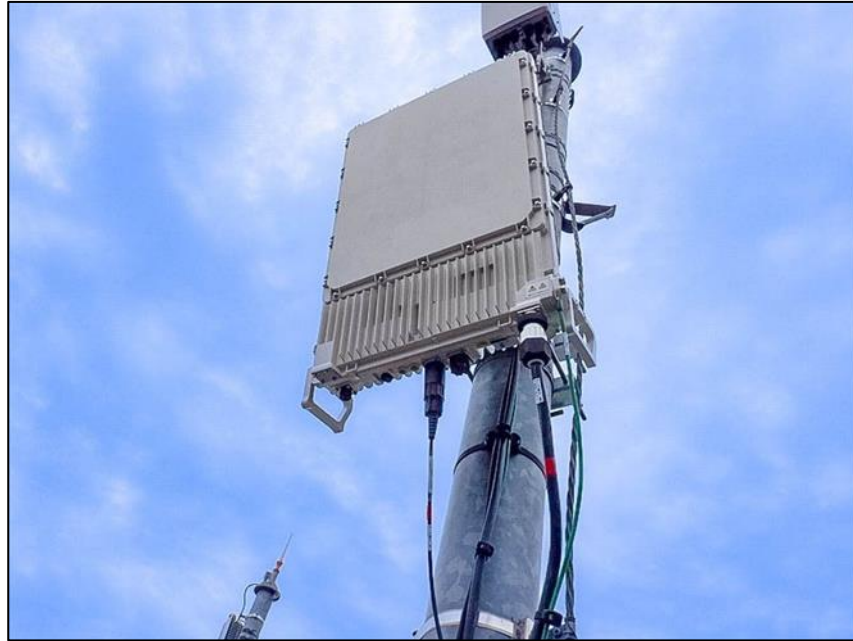
Figure 2-5 Open virtualized 5G base station commercially deployed by KDDI CORPORATION Source: Press release by KDDI CORPORATION
